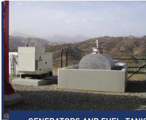
GENERATORS AND FUEL TANK
